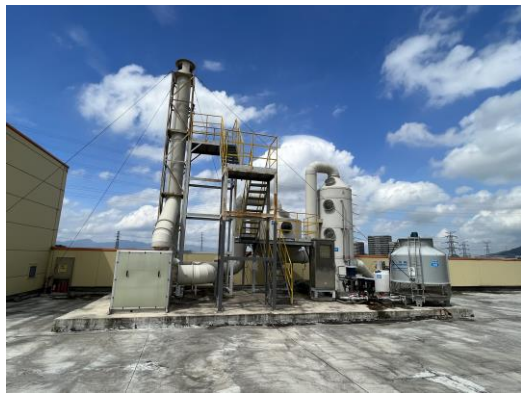
30TH 恶臭废气排放口 DA016
